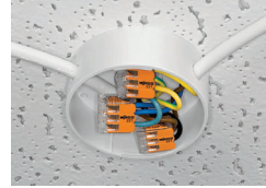
Lighting distribution in a ceiling canopy
